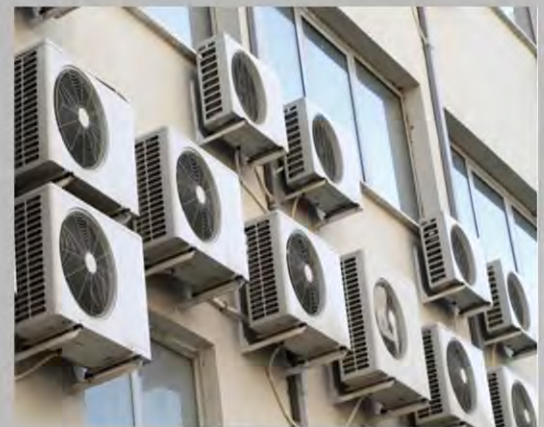
Unplanned Installations of Ac outdoor units which detracts the aesthetic look of a overall building & makes the maintenance difficult
